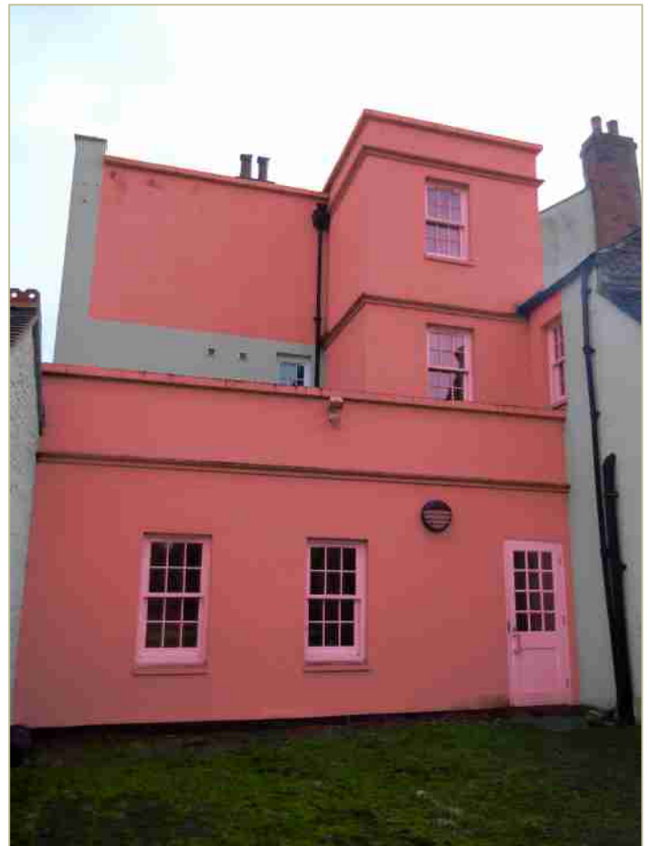
Figure 7.1, left, the western elevation during alteration work in c.2003. 7.2, right, the western elevation in 2014 with 2002 additions highlighted in red
